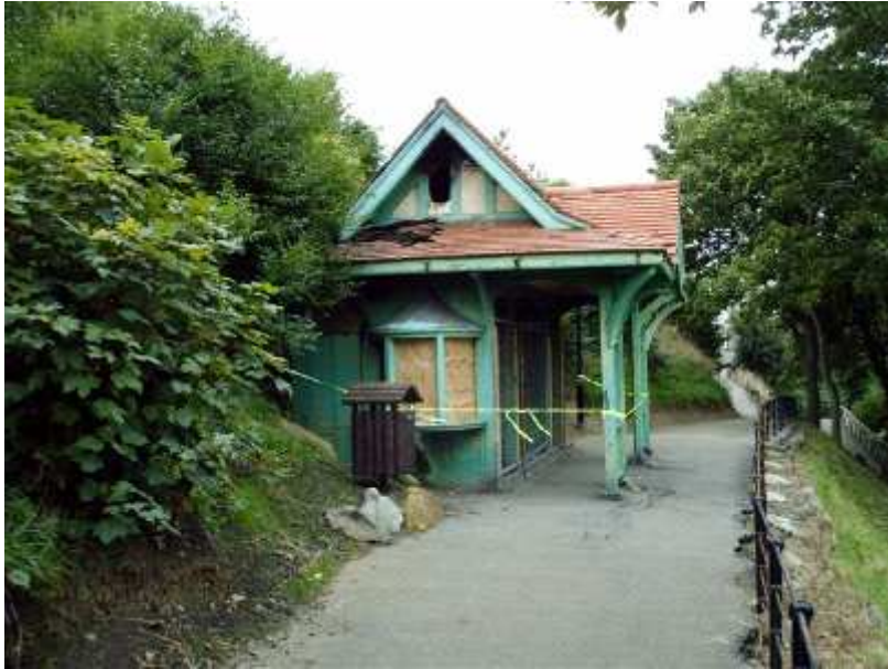
Before repair Shelter 12
